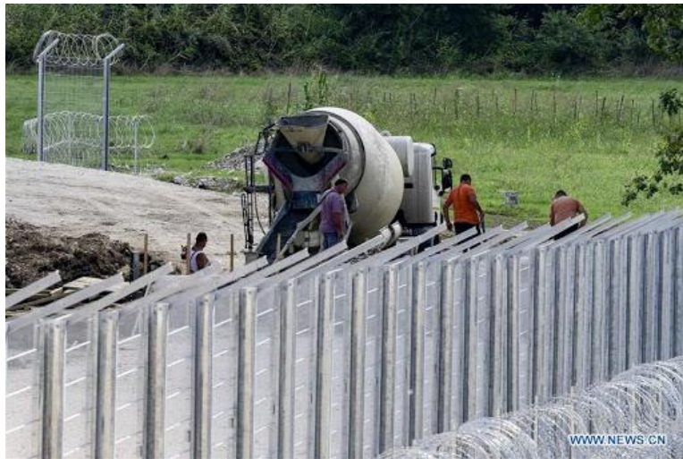
Figure 13: Fence between Turkey and Syria 71
