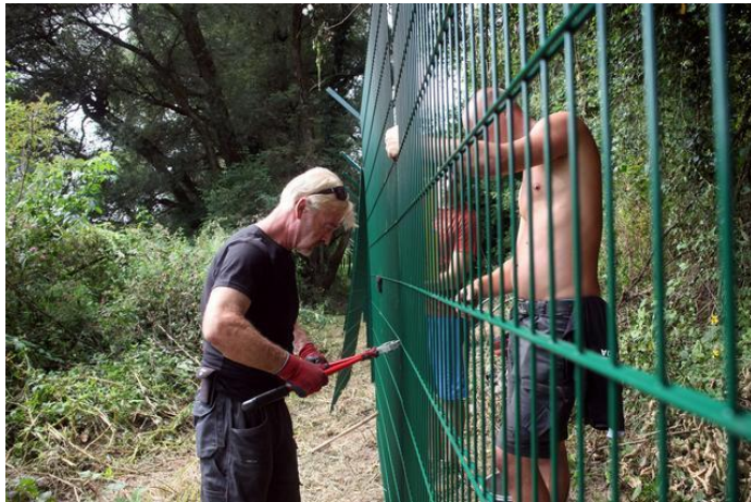
Figure 11: Workers build a fence in Slovenia near the River Kolpa in August 2019 64
